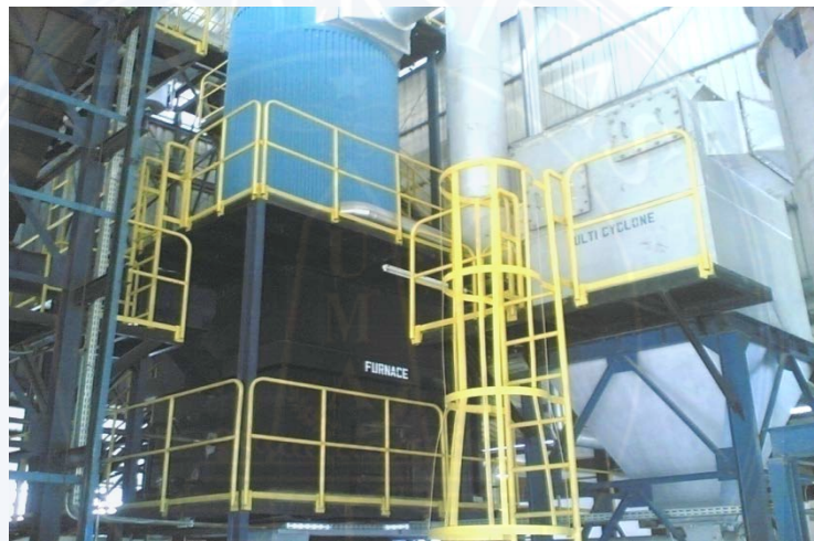
Gambar III-7. TOH (Thermal Oil Heater)
