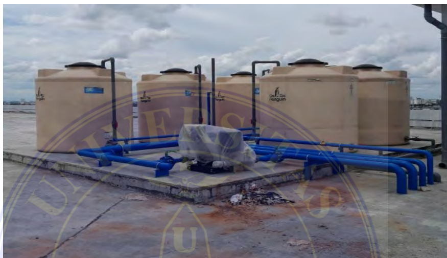
Gambar 5. Roof Water Tank (Rumah Sakit Regina Maris 2023)
