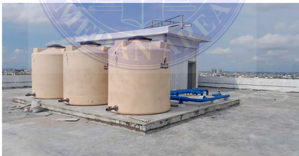
Lampiran 8. Tangki Air Atap / Roof Water Tank RS. Regina Maris Sebelah Kanan, 2023.
