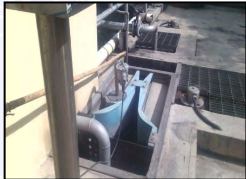
Gambar 4. Bak air terolah, up-flow filter, bak disinfektasi
