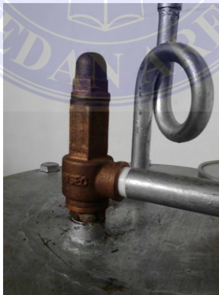
Gambar 2.11. Safety Valve ( katup pengaman )
