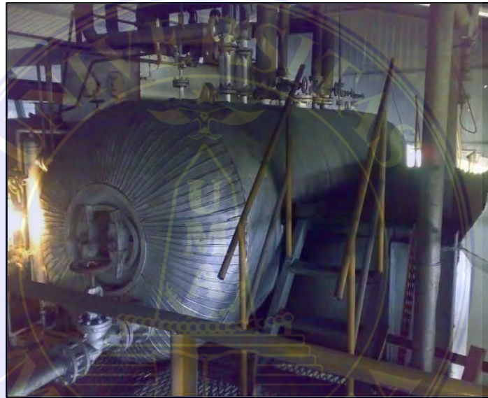
Gambar 2.8 Steam Boiler Drum
