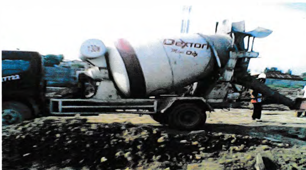
Gambar 3.1 Concrete Mixer (Readymixed)
