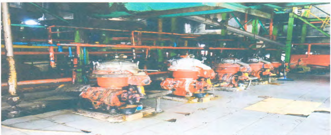
Gambar 13. Oil Purifier (sumber = Tim PKL di Kebun PTPN IV Unit Tinjowan 2019).
