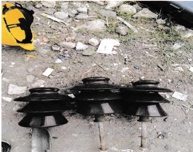
Gambar 3.1 Gangguan akibat Isolator Flash Over
