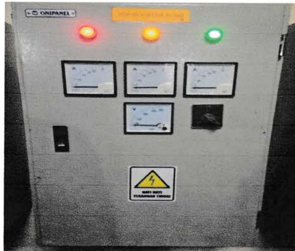
Gambar 3.3 : Panel Booster Pump di GMP
