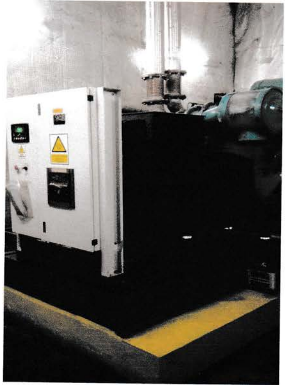
Gambar (e): Genset 800KVa GMP
