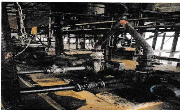
Gambar 3.26 Oil Transfer Pump
