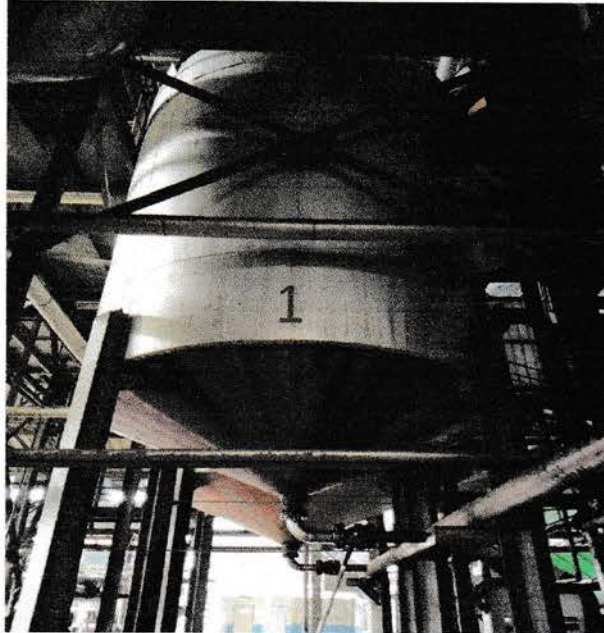
Gambar 3.16 Sand Trap Tank
