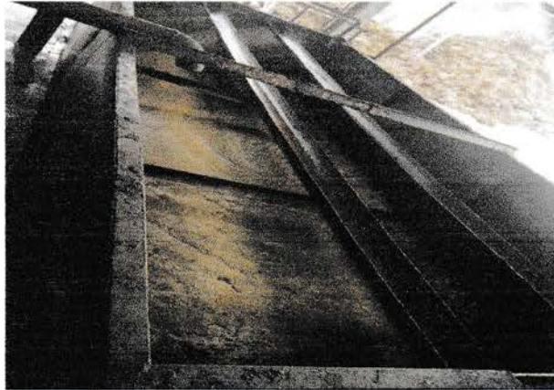
Gambar 3.18 Crude Oil Tank
