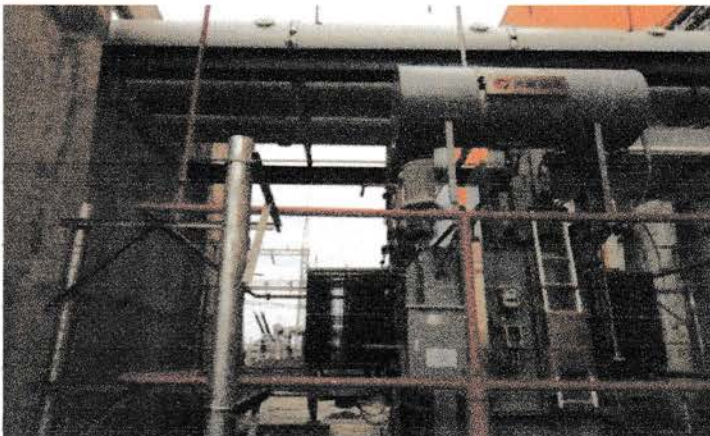
Gambar III. 10 : Trafo (transformator) AUT ( Auxularry unit transformer )
