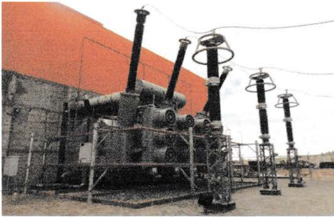
Gambar III. 9 : Trafo (transformator) GT ( Generator transformer )
