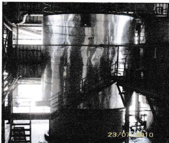
Gambar 3.7 Continuous Settling Tank
