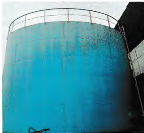
Gambar 3.38 Feed Water Tank
