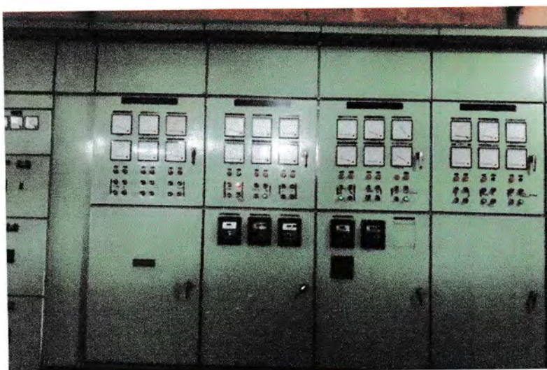
Gambar 3.42 Panel Distribusi Tenaga Listrik
