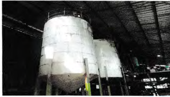
Gambar 3.52 Continous Settling Tank (CST)
