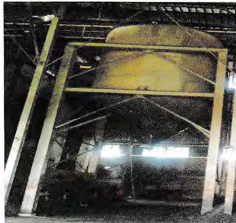
Gambar 3.32 Bunker Inti Sawit
