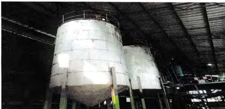
Gambar 3.17 Continous Settling Tank (CST)
