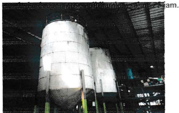
Gambar 3.52 Continous Settling Tank (CST)
