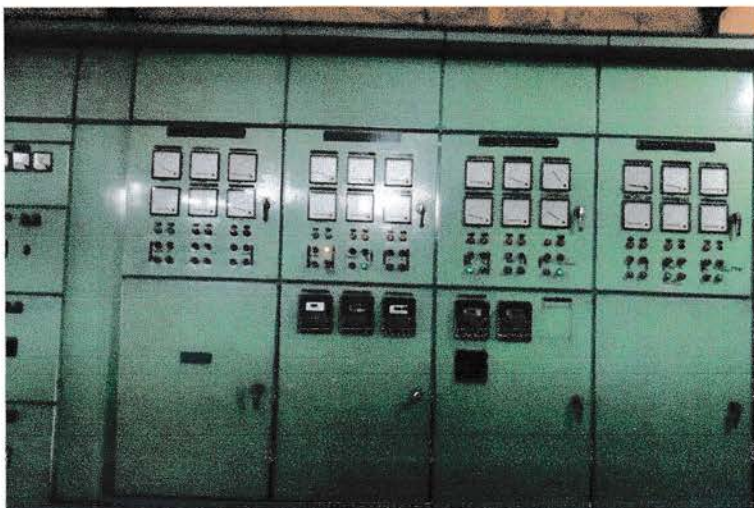
Gambar 3.42 Panel Distribusi Tenaga Listrik
