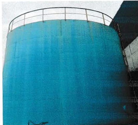
Gambar 3.38 Feed Water Tank
