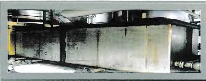
Gambar 3.25. Diluted Crude Oil Tank (DCO Tank)
