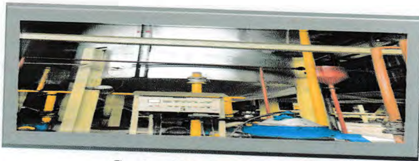
Gambar 3.28. Clean Oil Tank
