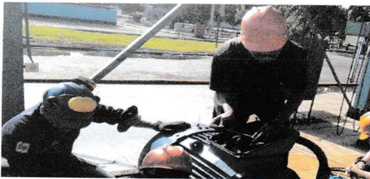
Gambar 3.4. Buka Cover terminal motor 380 V
