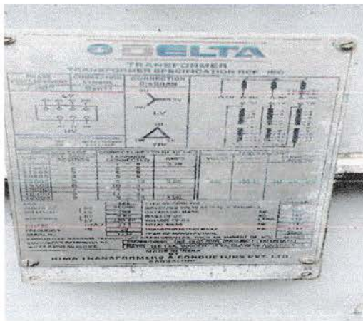
Gambar 2. 18 : Nameplate transformator PS
