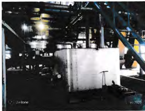
Gambar 3.19 Crude Oil Tank
