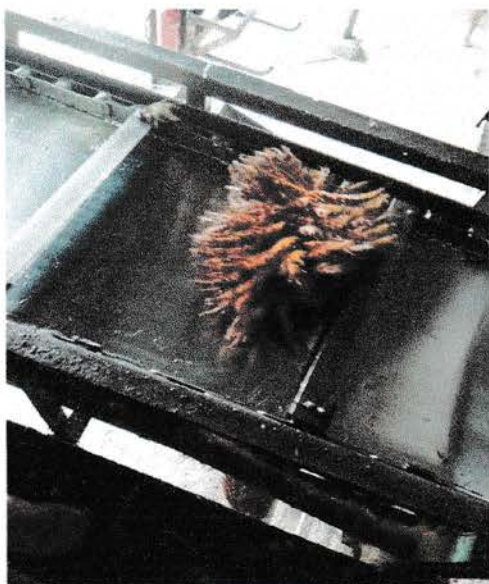
Gambar 3.13. horizontal empty bunch conveyor
