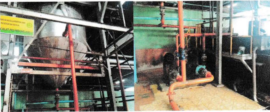
Gambar 3.16.m. sludge tank, preelener cyclone dan pump sludge buffer tank
