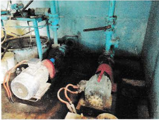
Gambar 4.1.1 raw water pump
