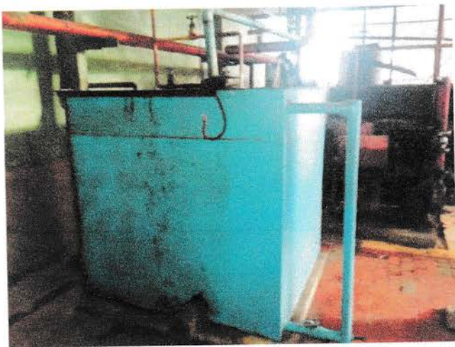
Gambar 3.16.1. hot well tank dan pump
