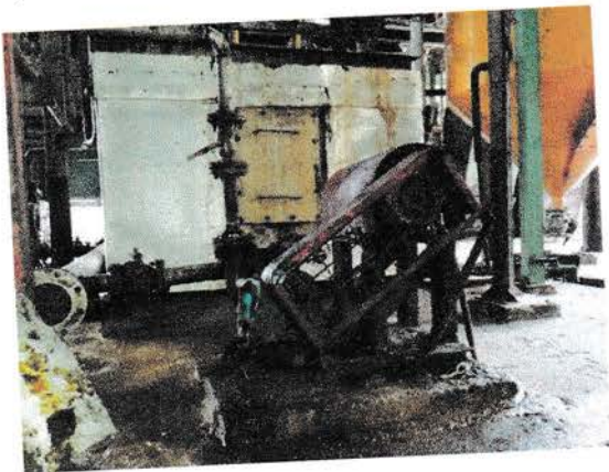
Gambar 3.16.b. tangki pompa minyak kasar (crude oil tank pump)
