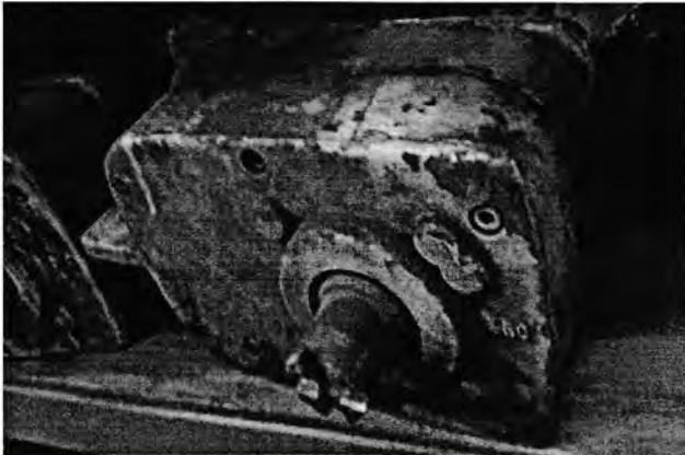
Gambar 4.1 Gearbox Overhead Crane.
