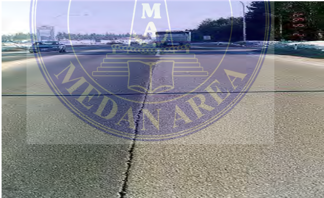
Gambar 2.3.5 Retak Sambungan Pelebaran ( Joint Reflection Cracking )
