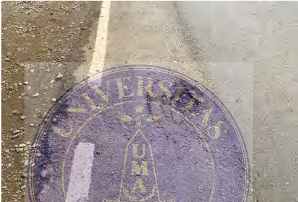
Gambar 2.3.4 Cacat tepi perkerasan ( Edege cracking )
