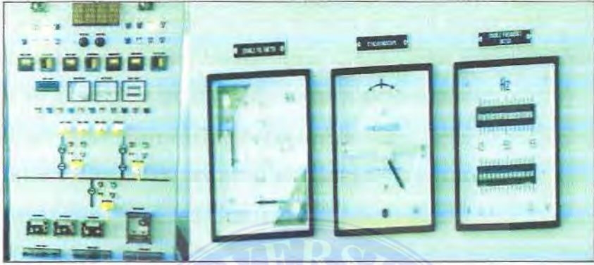
Gambar 4.23. Panel Sinkronisasi Ke PLN Di Biogas Plant PT. Agro Muko Palm Oil Mill
