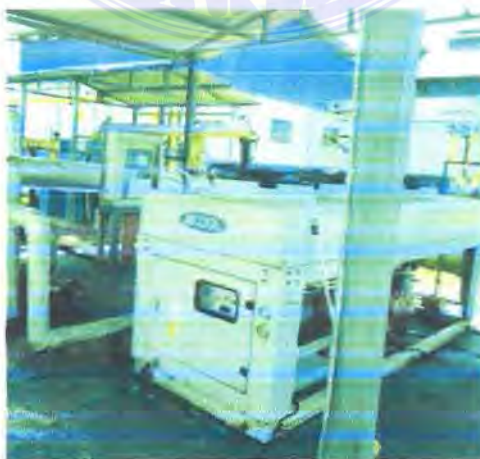
Gambar 4.18. Dehumidifier Biogas ( Chiller )
