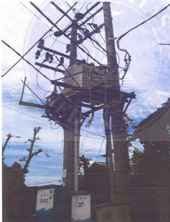
Gambar 2. 8 Gardu Transformator Distribusi
