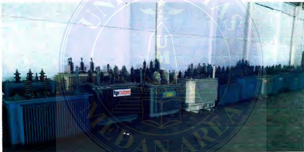
Gambar 2. 1 Trafo Distribusi 20 KV
