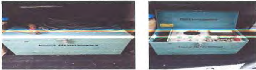
Gambar 3 2Motor over load relay dan circuit breaker
