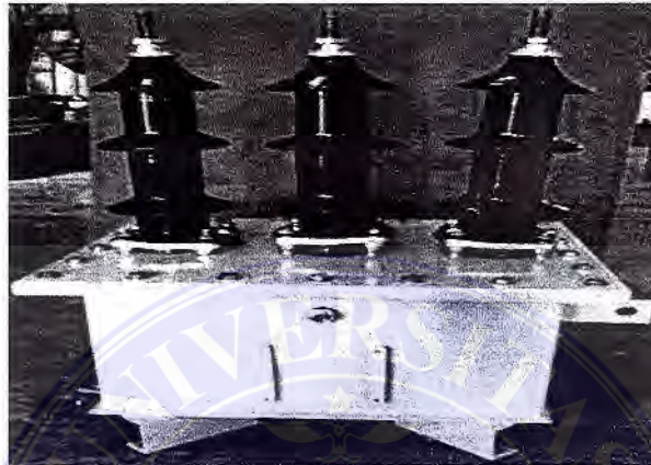
Gambar 2.8: Potential Transformer (PT)
