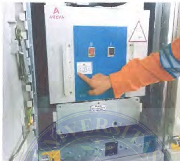
Gambar 11. Kubikel Incoming 20 kV
