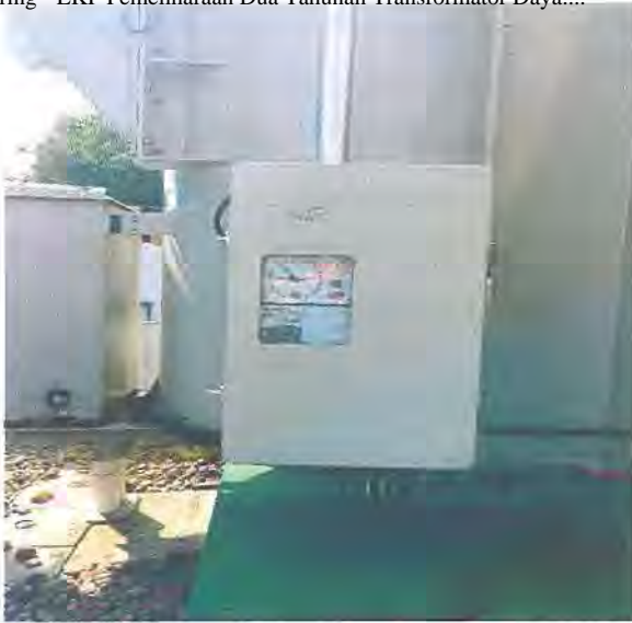
Gambar 7. Indicator Transformator Daya
