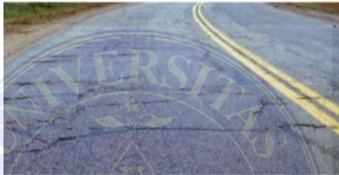
Gambar 2.4. Block Cracking Sumber : Dirjen Bina Marga 2017
