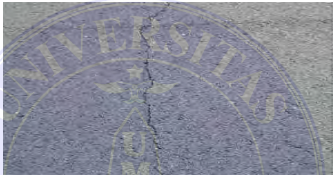
Gambar 2.11 Longitudinal and Transverse Cracking Sumber : Dirjen Bina Marga 2017
