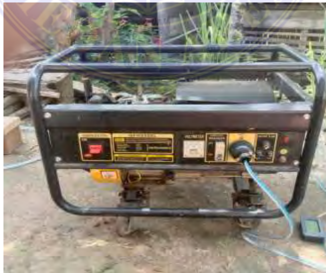
Gambar 3. 5. Generator Set Bensin
