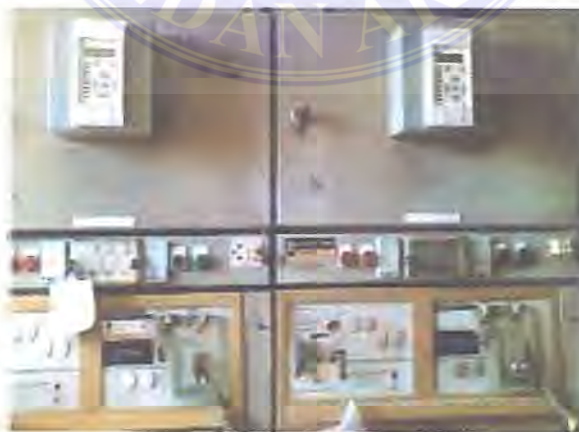
Gambar 3.6: Circuit Breaker Out
