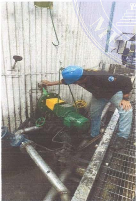
MENGAMATI LEVEL SWITCH
