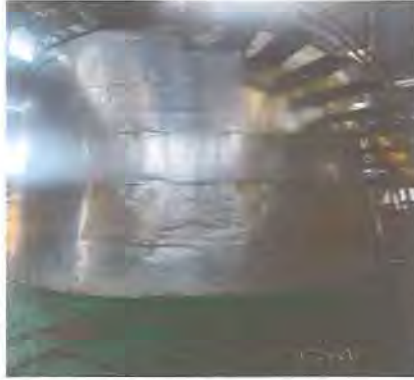
Gambar 3.14 Continuous Settling Tank
