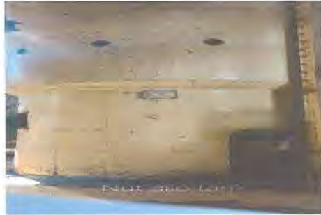
Gambar 3.23 Nut Silo Tank
