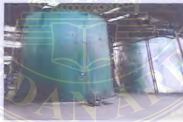
Gambar 3.34 Feed Water Tank
