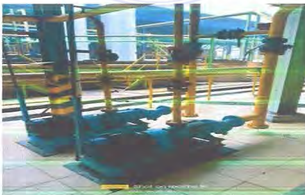
Gambar 3.6. Oil Pump final Transfer
