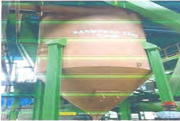
Gambar 3.5. Sand Trap Tank
