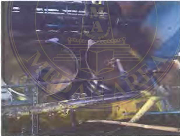
Gambar 3.14 Sludge Tank dan Oil Tank
