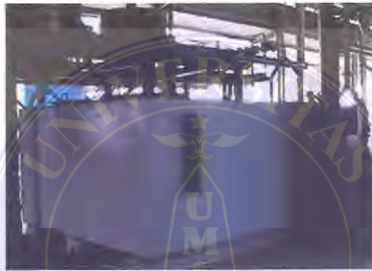
Gambar 3.13. Crued oil Tank
