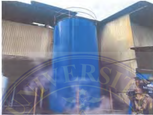
Gambar 3.21 Feed Water Tank
