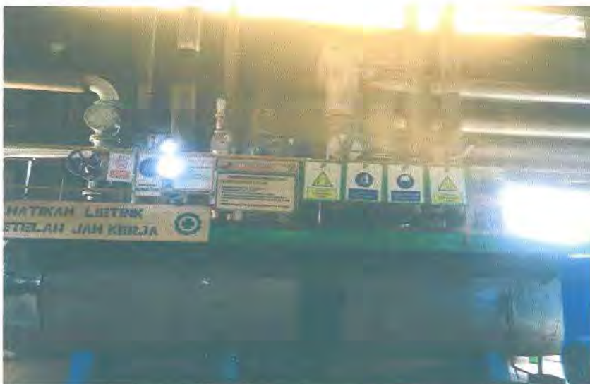
Gambar 3.45. Back Pressure Vessel
