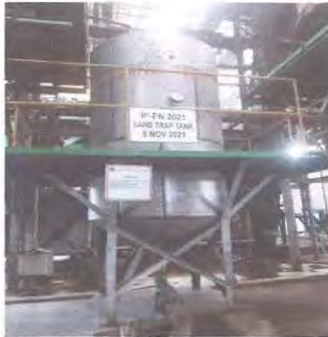
Gambar 3.26. Sand Trap Tank
