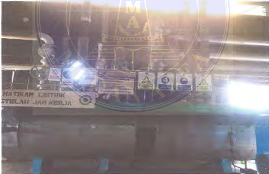
Gambar 3.46. Back Pressure Vessel
