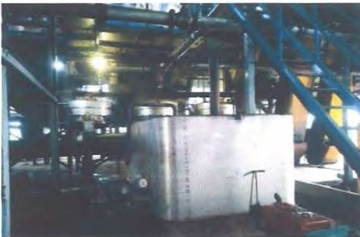
Gambar 3.19 Crude Oil Tank
