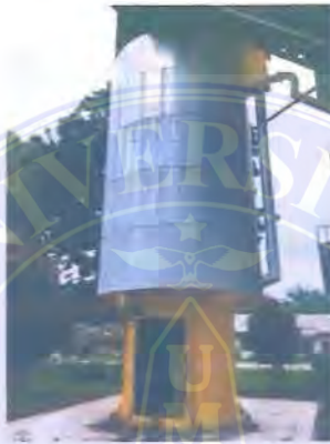
Gambar 3. 15 Continuous settling tank
