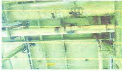
Gambar 3.30 Crude Oil Gutter
