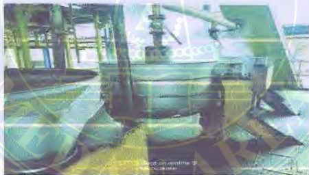
Gambar 3.31 Oil Vibre Separator
