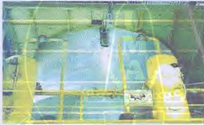
Gambar 3.33 Continious Settling Tank
