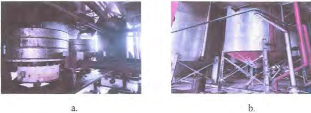
Gambar 3.11. (a) Oil Vibrating Screen (b) Crude Oil Tank
