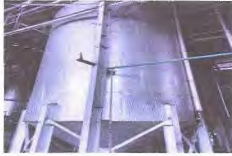
Gambar 3.12. Continous Settling Tank
