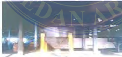
Gambar 3. 13 Sand Trap Tank
