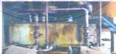
Gambar 3. 28 Crude Oil Tank
