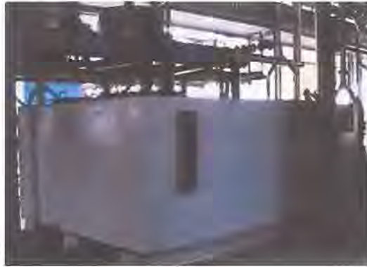
Gambar 3.13 Crude Oil Tank
