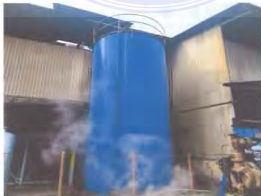
Gambar 3 21 Feed Waterr Tank
