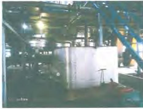
Gambar 3. 19 Crude Oil Tank
