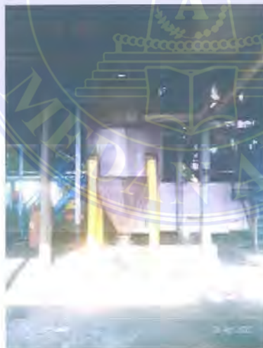
Gambar 3. 17 Sand Trap Tank
