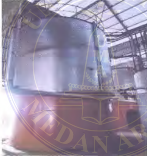
Gambar 3.19 Continuous settling tank
