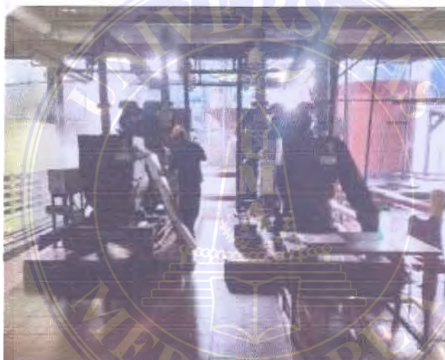
Gambar 3. 36 Mesin Diesel / Genset
