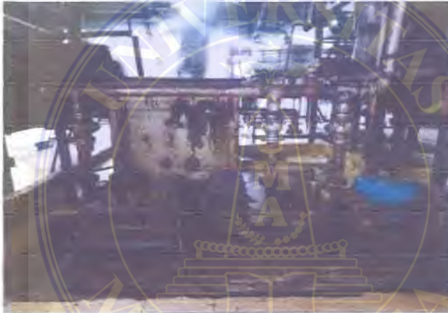
Gambar 3. 25 Crude Oil Tank
