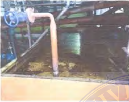
Gambar 3. 32 Sludge Drain Tank
