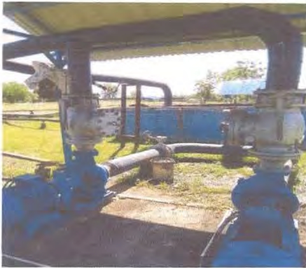
Gambar 3.5 Pump Mixing Tank Sumber : (Dokumentasi kerja praktik )
