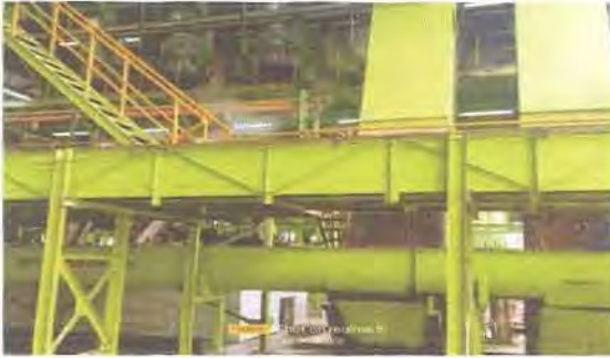
Gambar 30. Horizontal empty bunch conveyor
