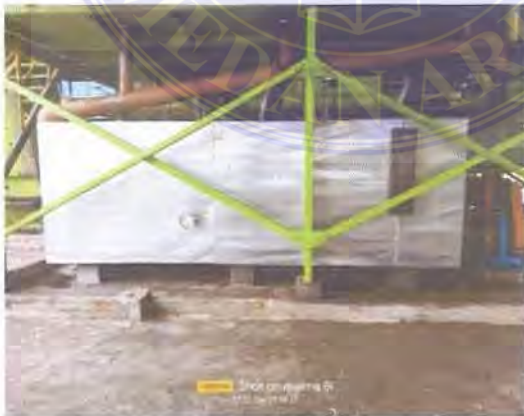
Gambar 33. Crude oil tank
