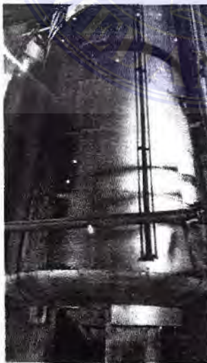
Gamabar 3.19 Sludge Tank
