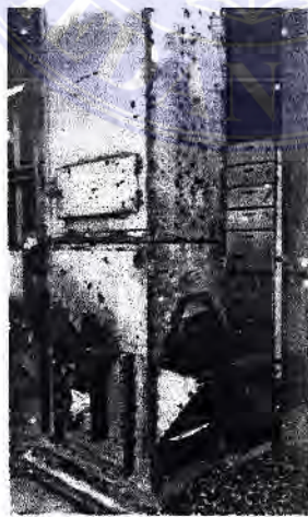
Gambar 3.30 Cracked Mixture Elevator
