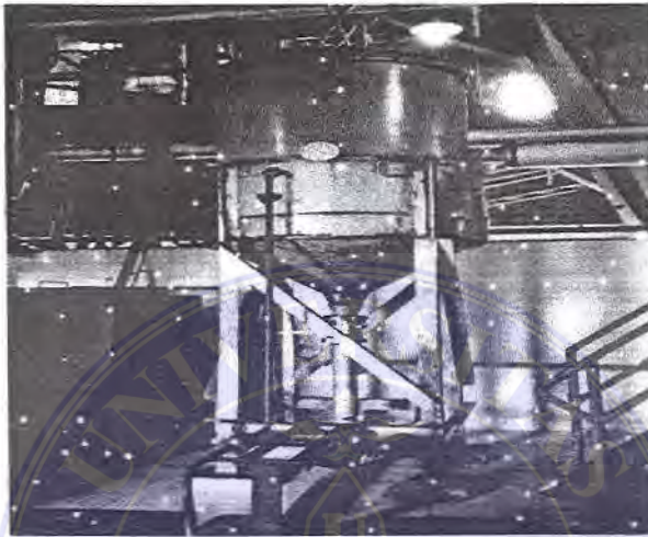
Gambar 3.11 Sand Trap Tank
