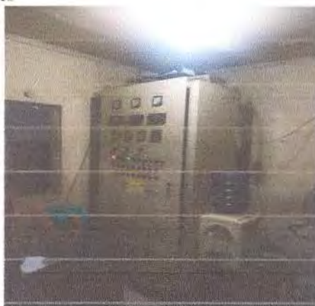
Gambar 3.15 Panel Kontrol Boiler
