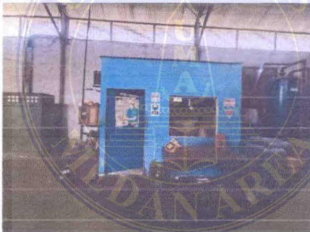
Gambar 3.14 Ruang Kontrol Boiler
