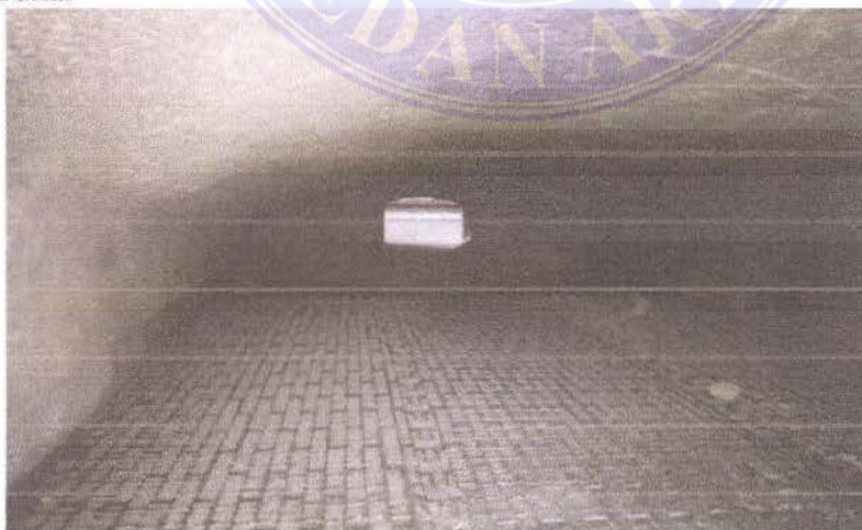
Gambar 3.9 Ruang Bakar Boiler
