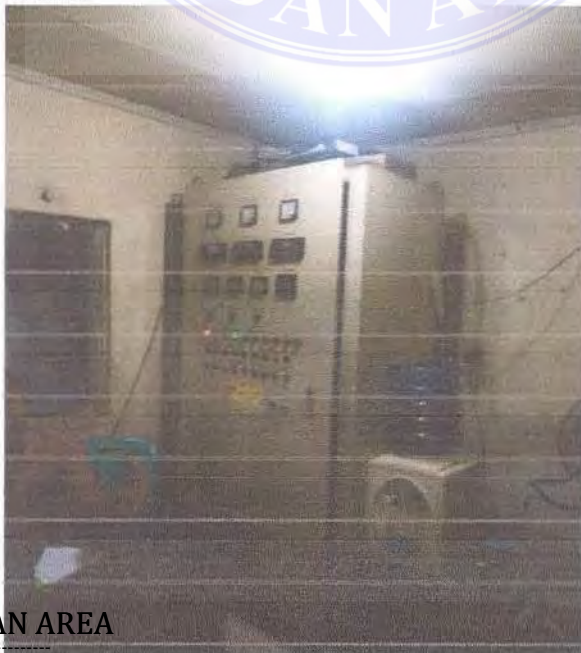
Gambar 3.15 Panel Kontrol Boiler
