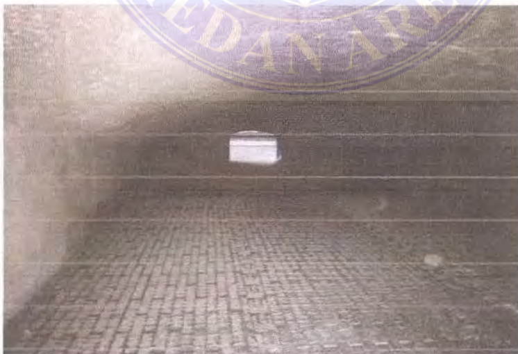
Gambar 3.9 Ruang Bakar Boiler
