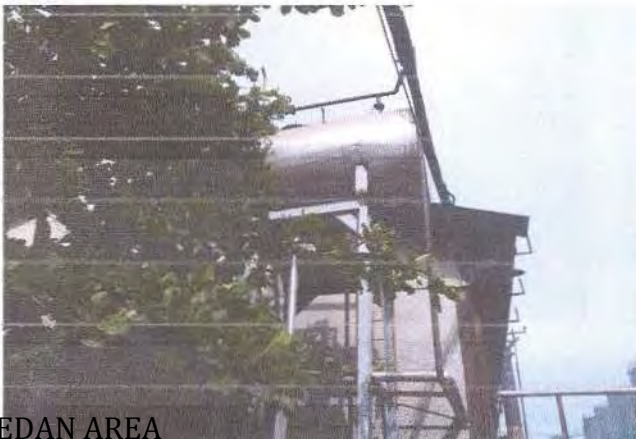
Gambar 3.18 Feed Water Tank
