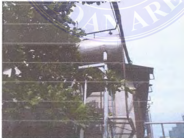
Gambar 3.18 Feed Water Tank
